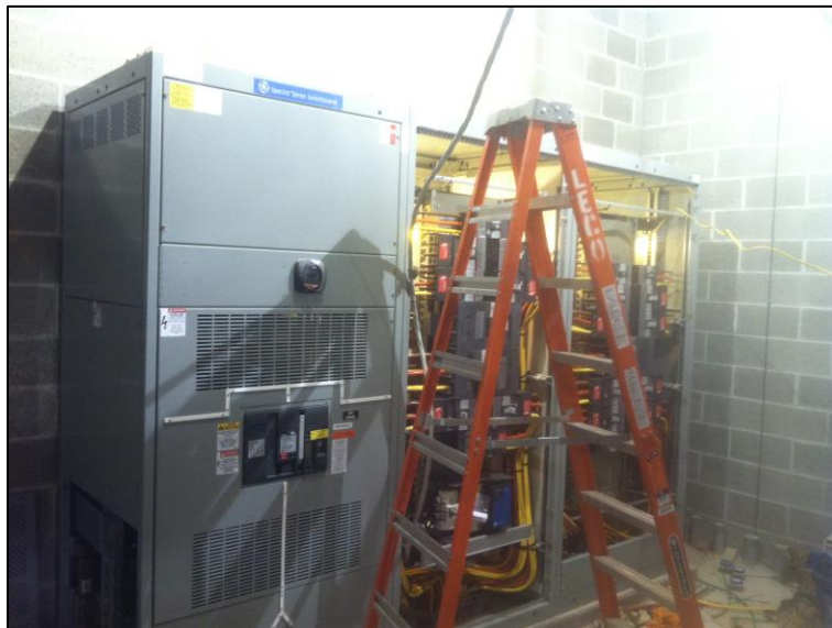
Figure 2: 3000A Main Switchboard (Property of Mascaro Construction)
