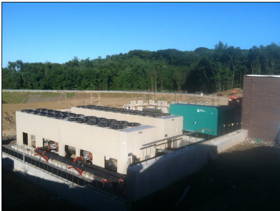
Figure 3: Chillers & Diesel Generator shown in Mech. Yard (Property of Mascaro Construction)
